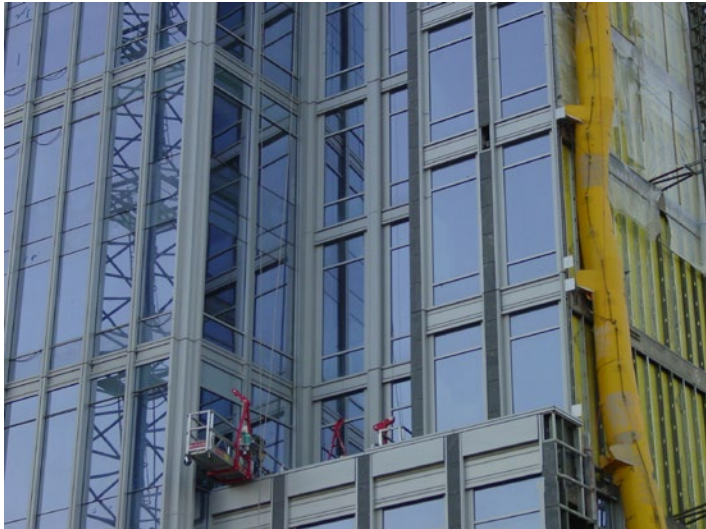
When completed, the new Pier 1 Center will employ approximately 94,440 linear feet of DOWSIL™ 756 SMS Building Sealant in joints between glass, stone and aluminum substrates. [Photo courtesy of CDC, Inc.]
