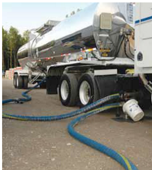
Dow experts work with local distributors to help manage the logistics of delivery and installation. At SVSU, two 10,000-gallon shipments of DOWFROST Fluid were delivered and trucks emptied quickly and efficiently.
