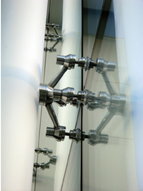
Figure 23: Crystal clear silicone adhesive tape is used in point bonding the glass units that gives un-interrupted, uniform & sleek facade design.
