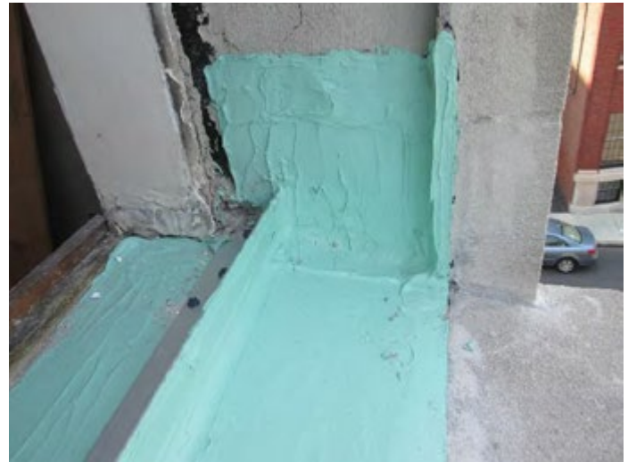
Figure 2: Liquid flashing installation at window opening – single material and installation operation. Image courtesy of Simpson Gumpertz & Heger – Waltham, Massachusetts.
