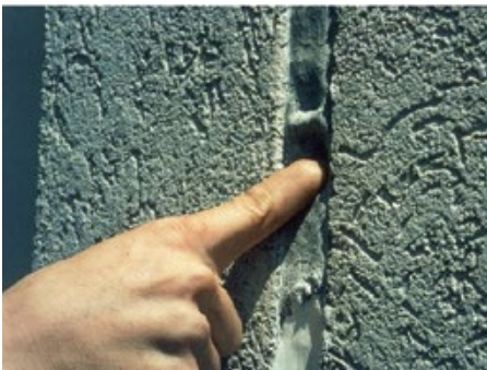
Polyurethane sealant cracking
