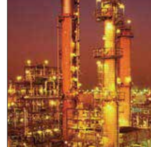
Process Heating and Cooling
