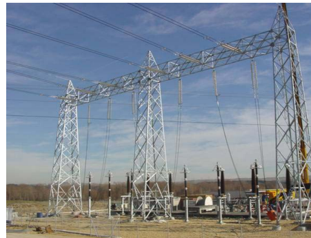
Figure 5: Overhead line cables transition station (400kV)
