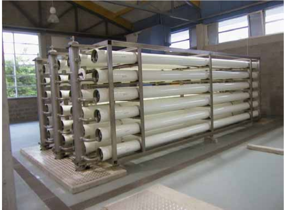
Pressure vessels housing reverse osmosis elements at the water treatment facility (Photo courtesy of Intermunicipal Water Company of the Veurne Region)
